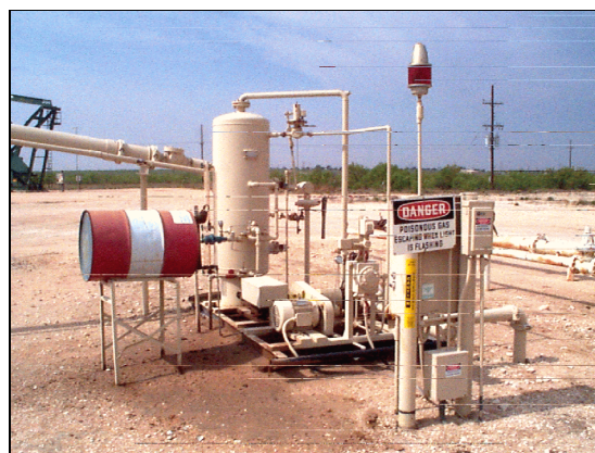
Figure 5. A vapor recovery unit.
